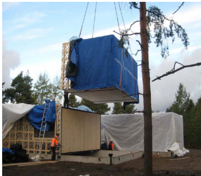
Figure 1. Prefabricated CLT-modules are fast to build on site (Pictures: Woodsolutions 2014 and Puumerkki 2014, Plan of action: Stora Enso).
