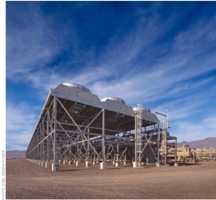
Stillwater Geothermal Plant in Nevada
